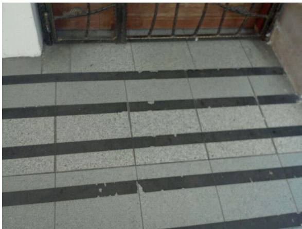
Image 4: Slippery epoxy lines
